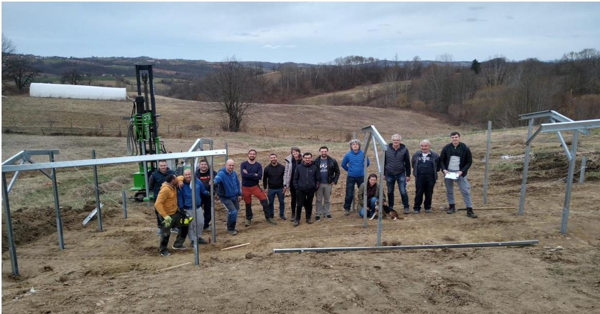
Photo: Installation of agrisolars on the Organela farm, Source: Elektropionir
